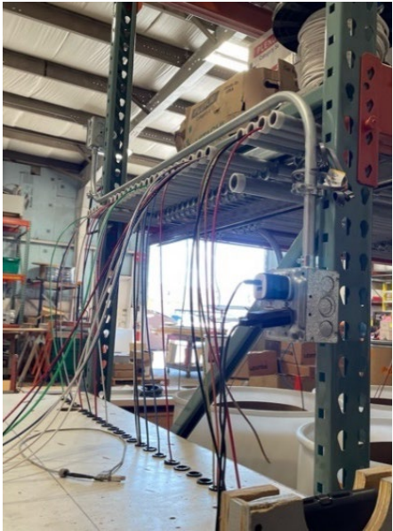
Image courtesy of Thompson Electric
